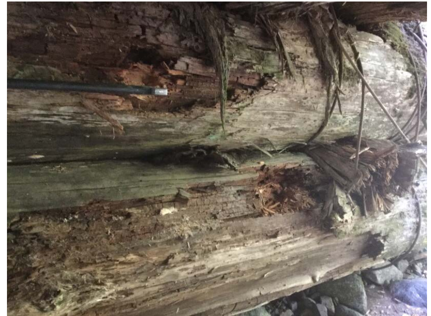
Cribs in poor condition, greater than 150mm sap rot
